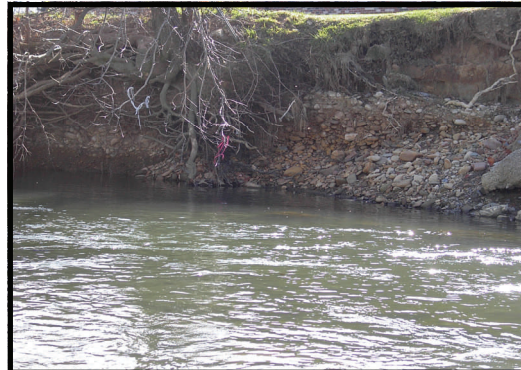
View of erosion and undercutting
