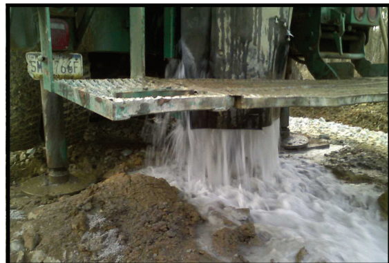
Flowing artesian well, producing 200+ gallons per minute.
